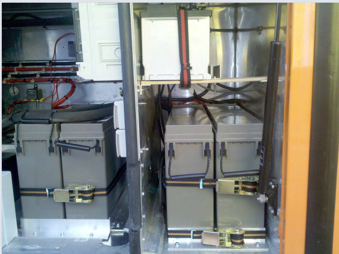
Foto 2: Vier Victron Telecom accu's.
